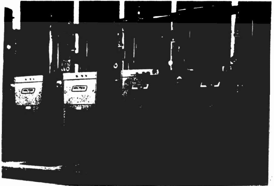
Multi-Pulse heating plants use individual, low-water content, smaller capacity boilers, such as this M-300 modular installation, where off-cycle losses are substantially reduced and dissipated heat from stored water is much less than large capacity, single input units.
